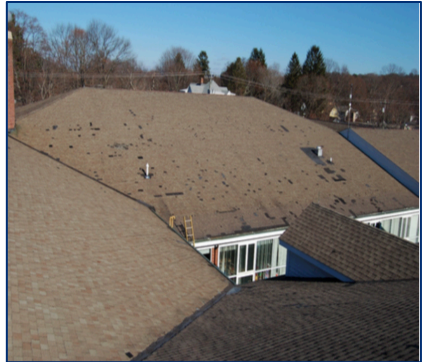
Numerous asphalt mastic patches
