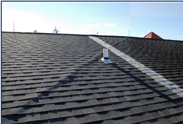
Failed GAF Shingles
